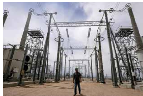
A workman stands outside, dwarfed by electrical substation technology. A massive substation at the coal-fired Intermountain Power Plant in Utah links the facility to transmission lines that deliver power to Southern California. A $2.65 billion project, just getting underway, will install facilities there to generate electricity from cleanly produced hydrogen.
