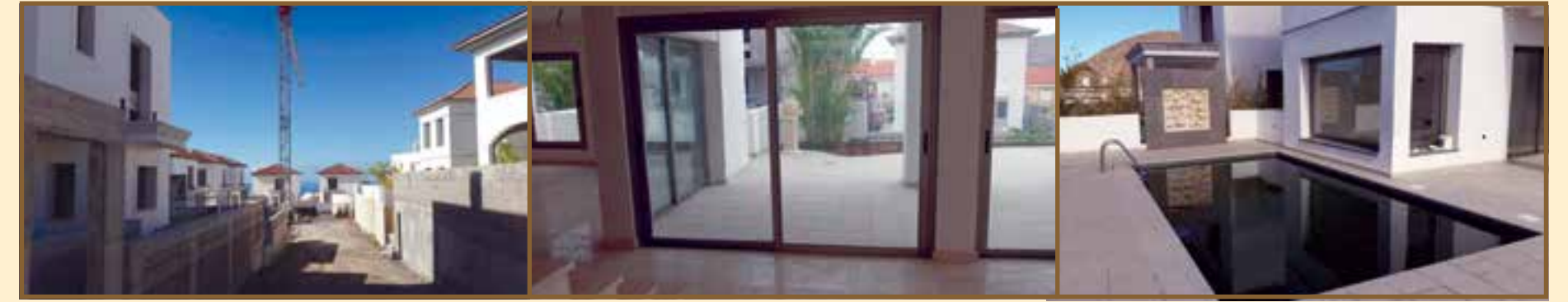
Photographs: Complex under construction, lounge and patio near completion and swimming pool.
