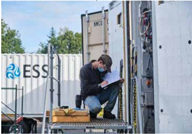
A worker at the ESS facility in Wilsonville, Oregon
