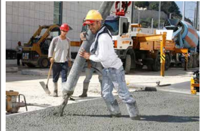
Dr Orr and his team carried out experiments to test the strength of concrete made with plastic
