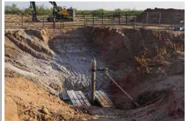
A decades-old, plugged and abandoned oil well at a cattle ranch in Crane County, Texas, in June 2021, when it was found to be leaking brine water
