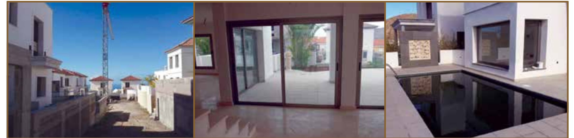
Photographs: Complex under construction, lounge and patio near completion and swimming pool.
